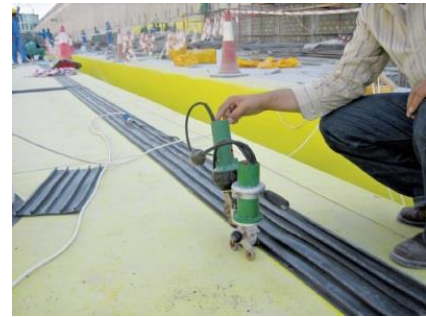
Waterbar welding onto membrane with Leister Triac Drive semi automatic heat welding device
