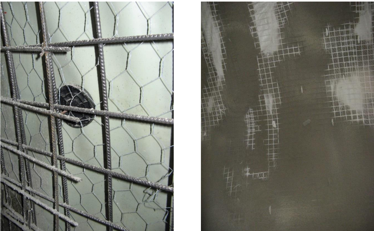
Figure 28: Spraying process over chicken wire and mesh fixed with a counter disc system
