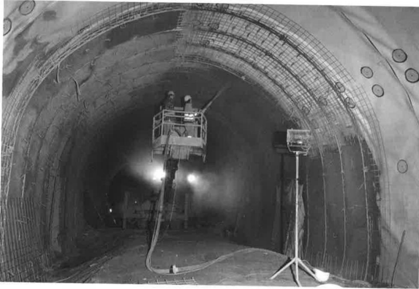
Figure 25: Over-spraying of felt laminated membrane, steel mesh kept in place with BA-Anchors
