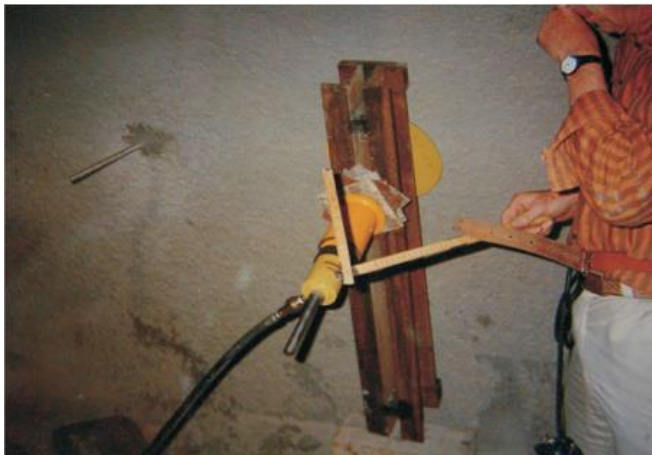
Figure 11: Flurlingen Tunnel / Switzerland, pull out test synthetic anchor with Sikadur 31 Epoxy adhesive, anchor steel screwed 130 mm into hard PVC shell
